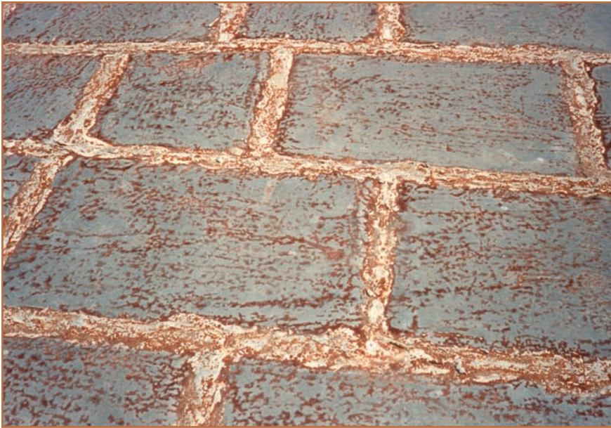
Photo 3: The owner of this roof off the coast of Maine complained that the lead was coming off his lead-coated copper. In actuality, “red lead” patina was forming.
