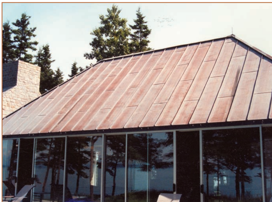
Photo 2: A new copper roof on a home in Charleston, SC, showed uneven weathering after the contractor “neutralized and washed down” the copper to remove residual flux.
