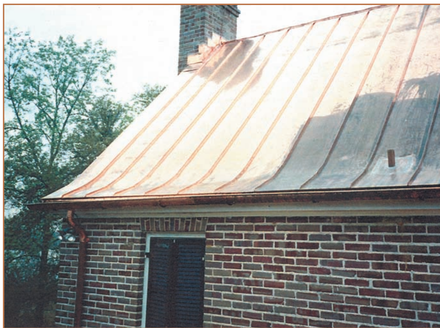
Photo 1: This Maryland residence shows normal but unusual weathering.
